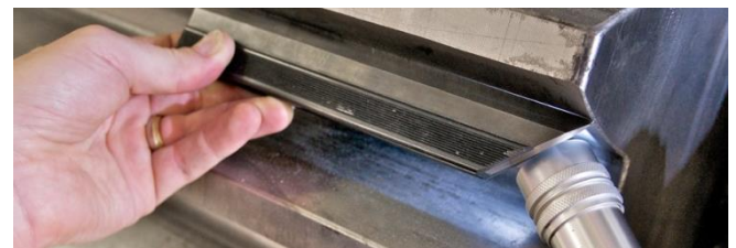
Wear inspection at the loaded flank of large tooth gearing
